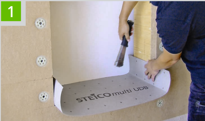
Applying the diffusion-open STEICO underlay STEICOmulti UDB as temporary weather protection until window installation
